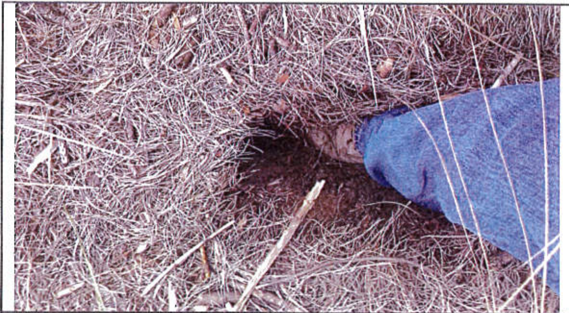
Photo 11: Slope erosion – northeast corner.
