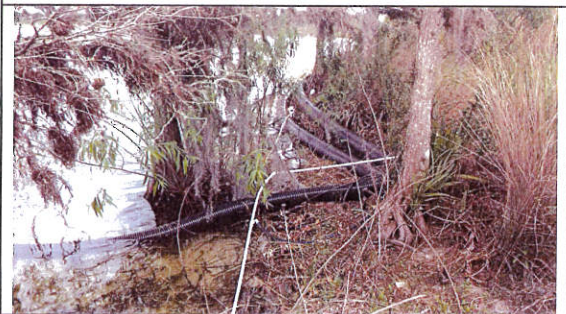
Photo 6: Exposed utilities due to slope erosion.
