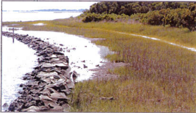
Figure 8a: Photograph of a Living Shoreline with a Toe Breakwater Structure. Photograph from the North Carolina Coastal Federation.
