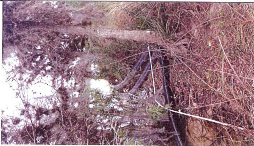
Photo 2: Exposed utility and irrigation pipes, northwest corner.
