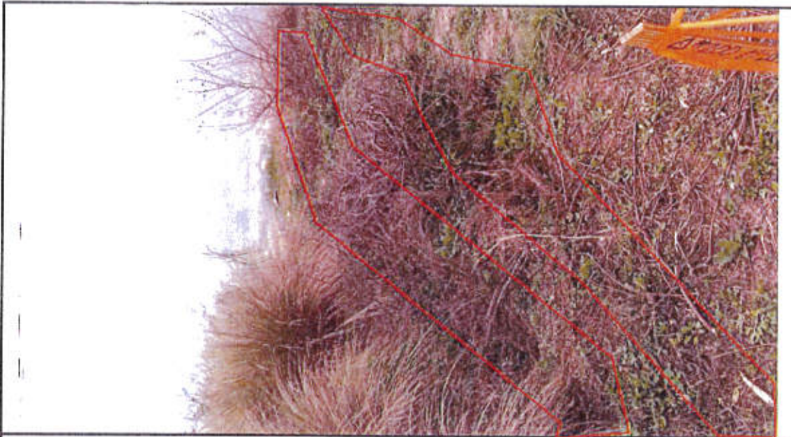
Photo 13: Slope erosion – northeast corner
