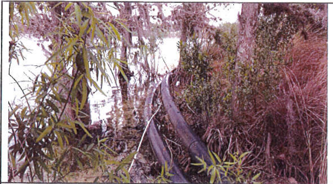
Photo 7: Exposed utilities due to slope erosion.
