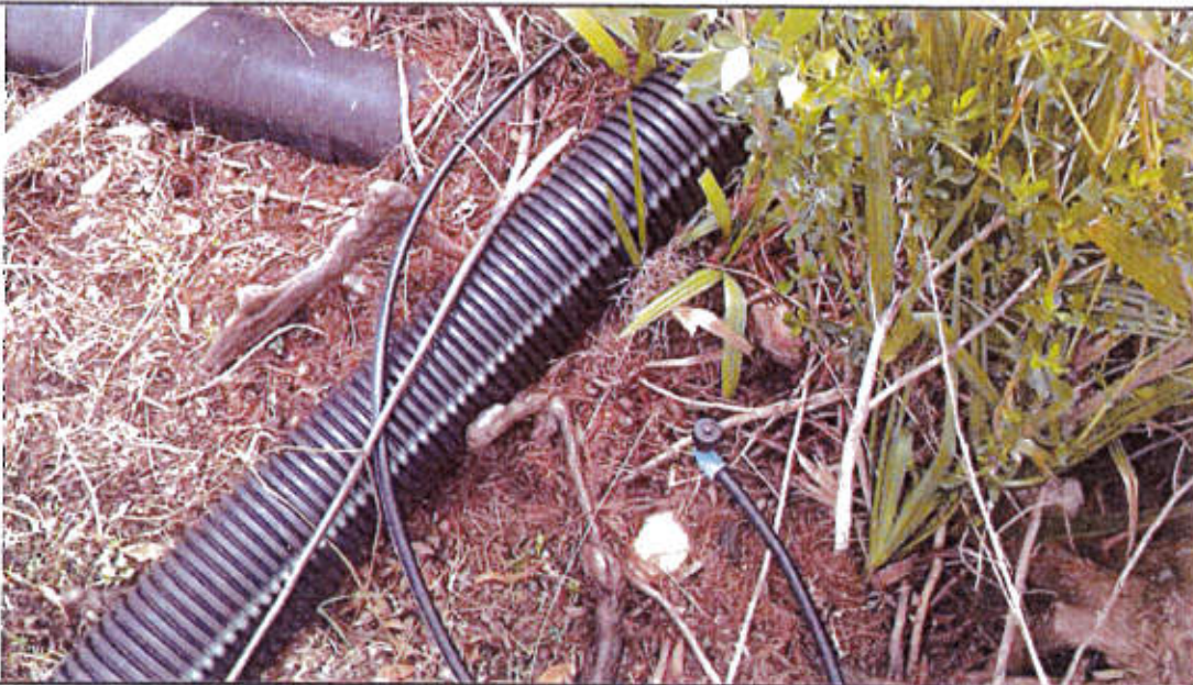
Photo 3: Exposed utility and irrigation pipes, northwest corner.
