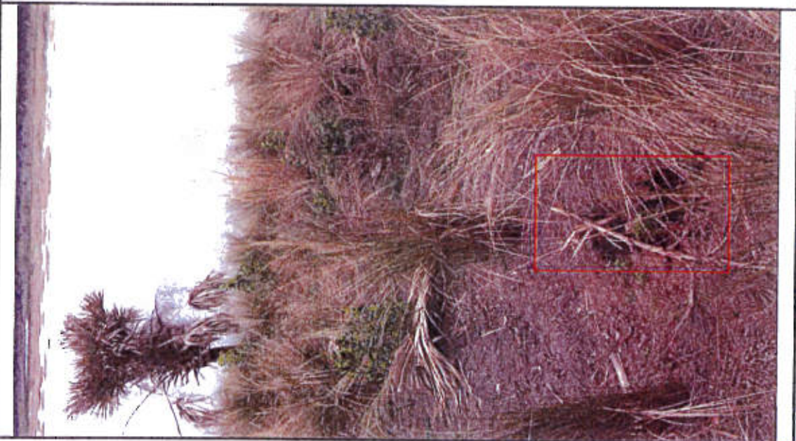
Photo 10: Slope erosion – northeast corner.
