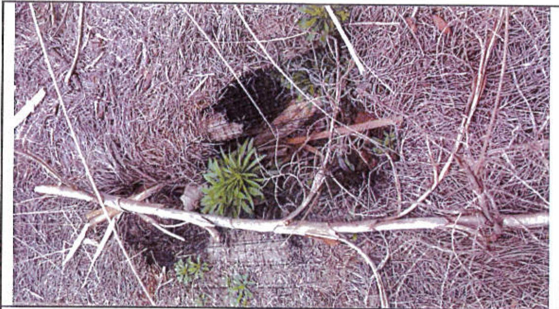
Photo 9: Slope erosion – northeast corner.
