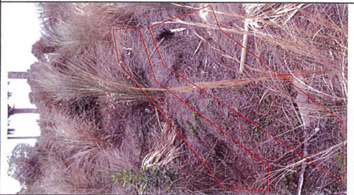
Photo 12: Slope erosion – northeast corner.
