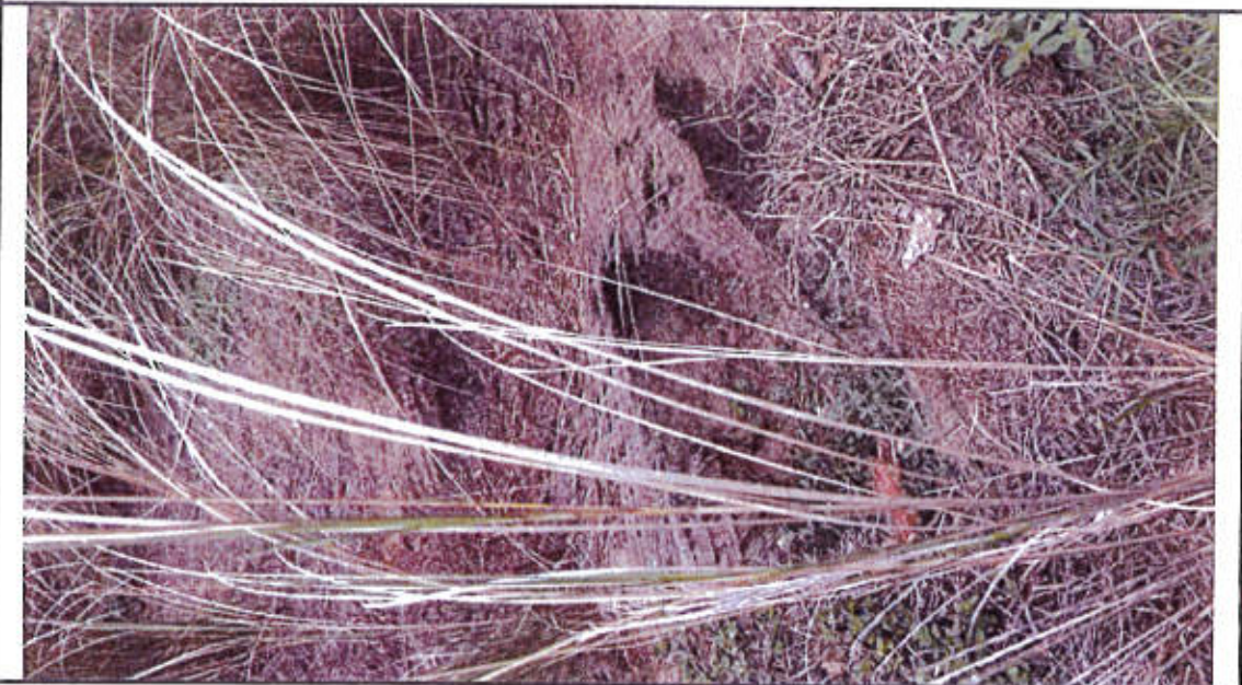
Photo 14: Slope erosion – northeast corner.
